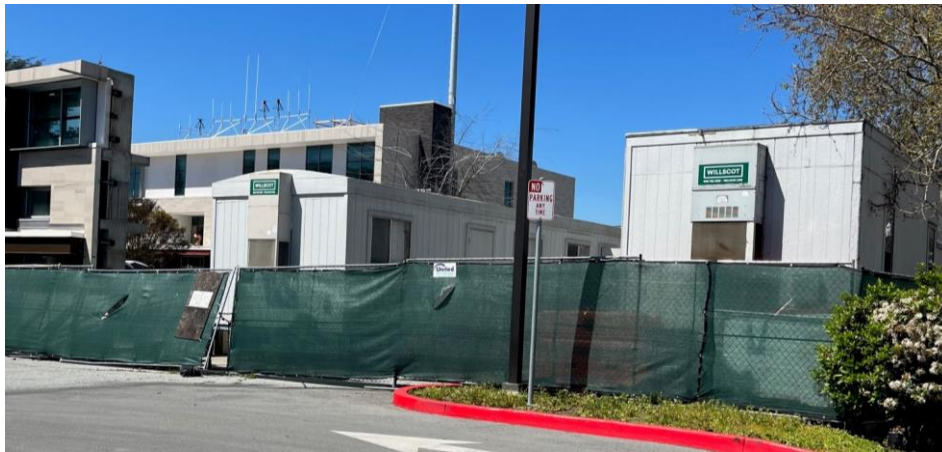
WSC modular facilities utilized in the construction of the Palo Alto Public Safety building.
